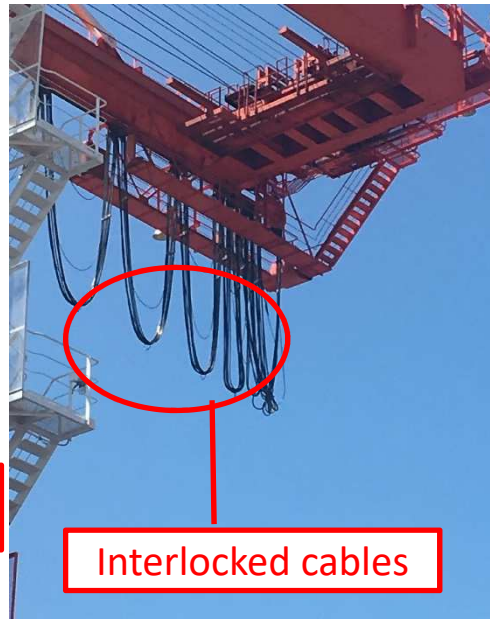
Damaged insulation coating
